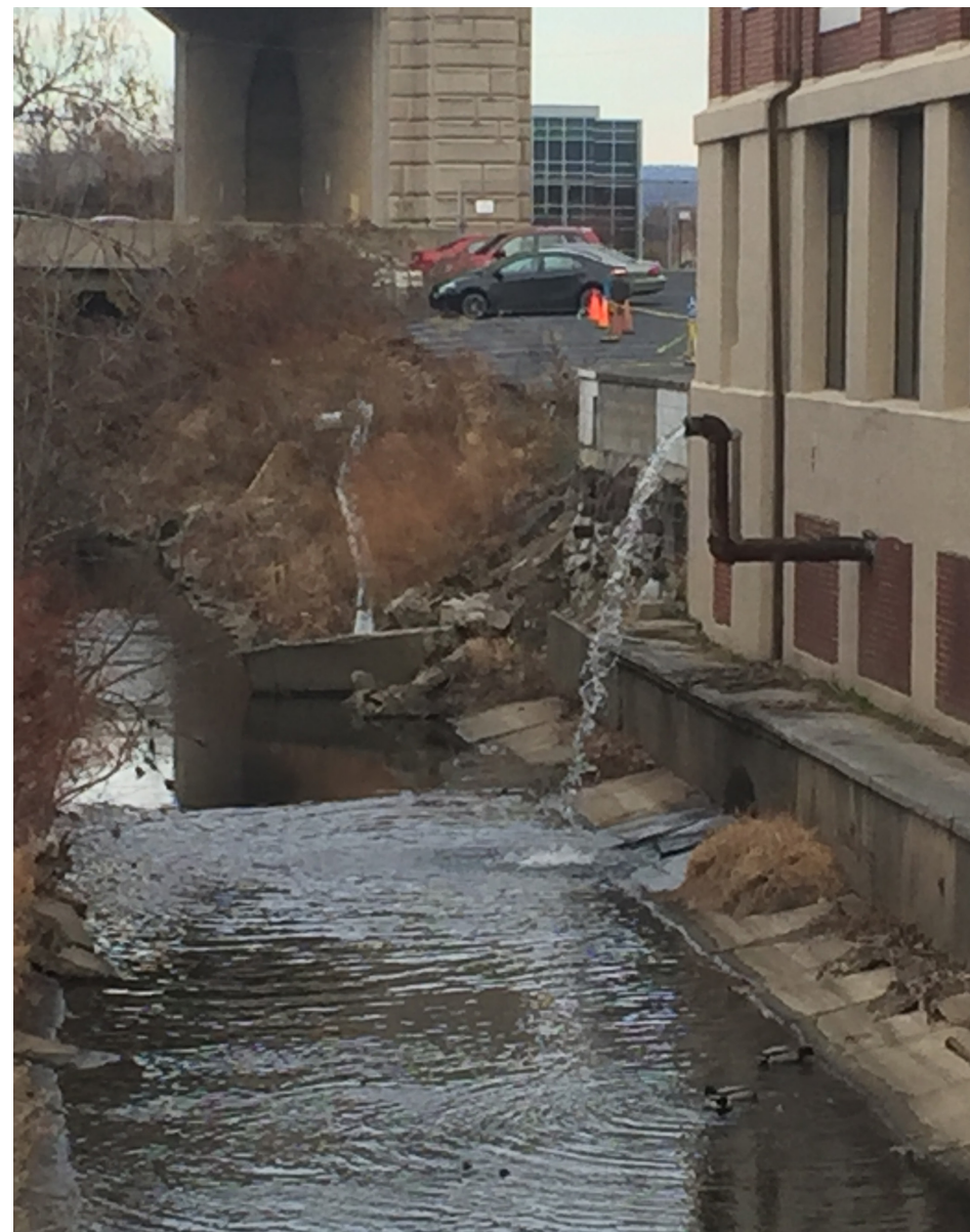
Urban Development Adjacent to and Deterioration of Modified Stream Channel
