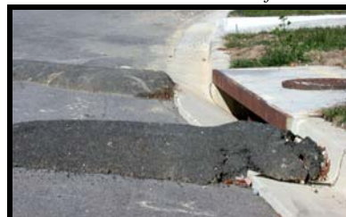
Asphalt barrier protects storm drain inlet from inputs of sediment
