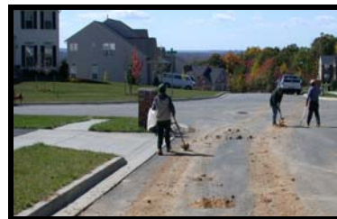
Cleaning up sediment from construction sites at the end of each day helps prevent sediment from leaving the site
