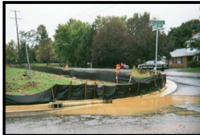
This failing silt fence allows muddy runoff to flow from the site
