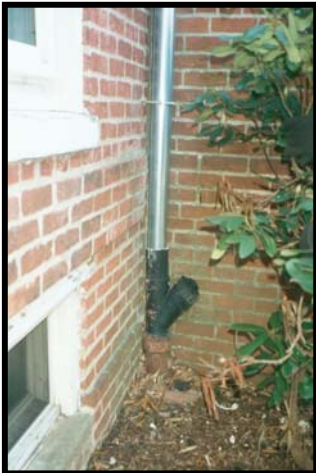
Downspout directly connected to stormdrain system
