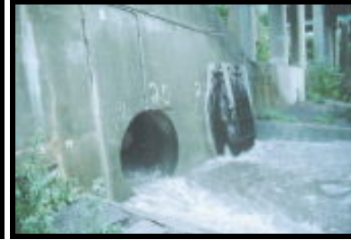
Combined sewer overflows discharge untreated wastewater to the stream when treatment plants are at capacity
