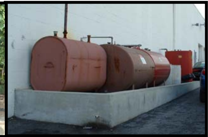
Motor oil storage containers with secondary containment berm
