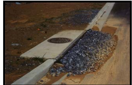
Poor inlet protection allows sediment to enter the storm drain
