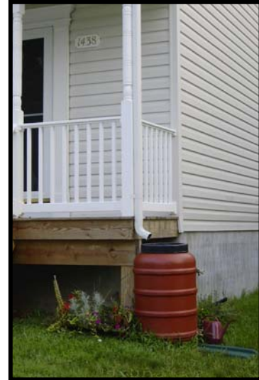
Disconnection to rain barrel
