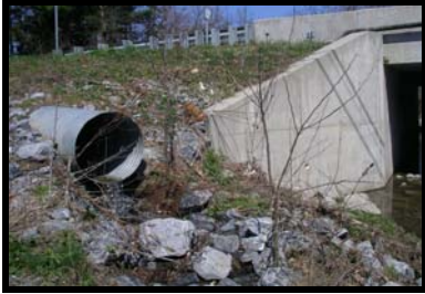
Urban runoff is transported through storm sewers and outfalls directly to this tributary of Paxton Creek
